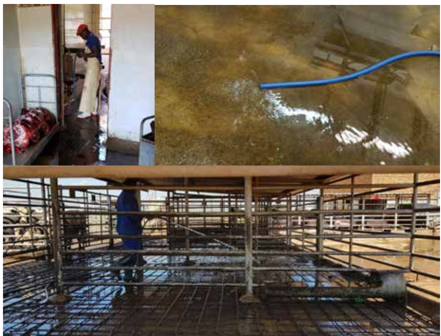
FIGURE 6: PIPING USED FOR RINSING/MANUAL CLEANING
