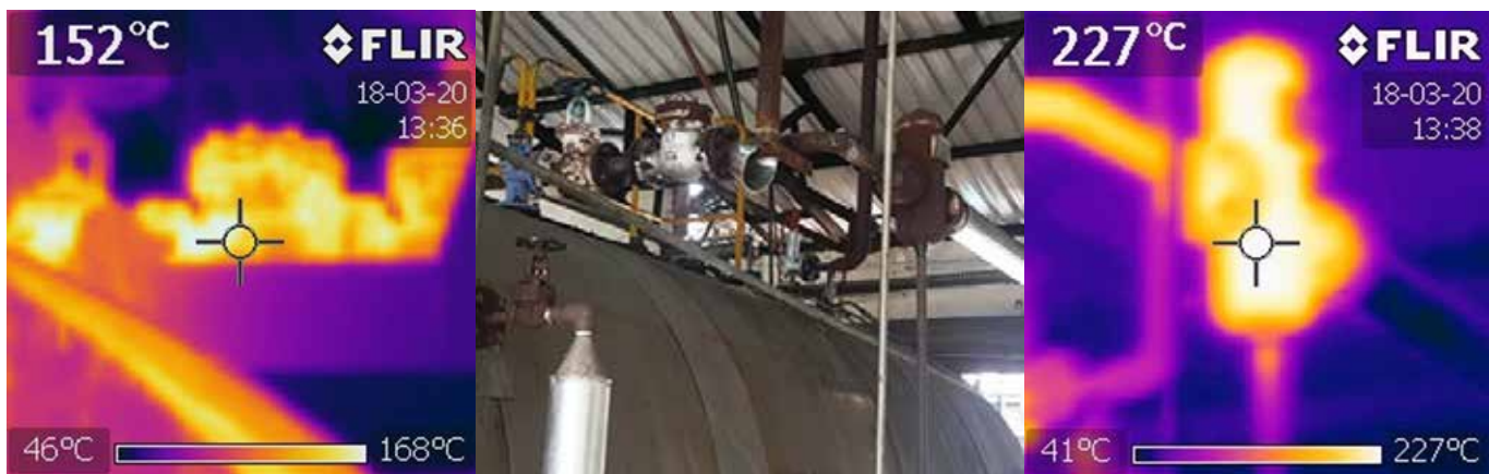
FIGURE 38: RADIATION LOSS PICTURES ON STEAM LINES
