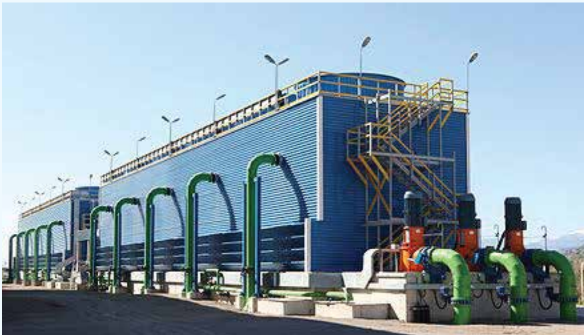
Figure 5-27: Industrial Cooling Towers for a Power Plant
