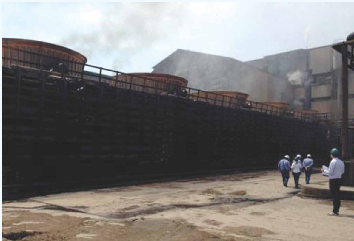
Figure 5-26: Cooling Tower from a Mexican Sugar Mill
