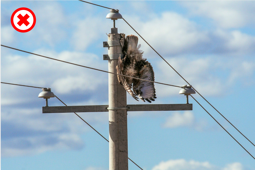
High Risk Structure
