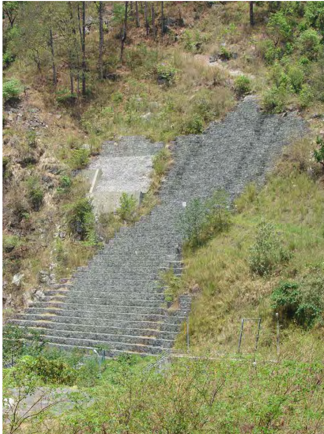
Remedial works to prevent landslide on unstable ground at Khimti 1 intake structure
