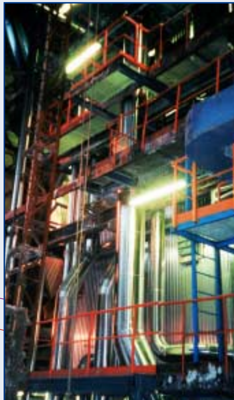
In Estonia, IFC supported the installation of a new recovery boiler to improve efficiency, emissions, and safety by Horizon Pulp and Paper.
